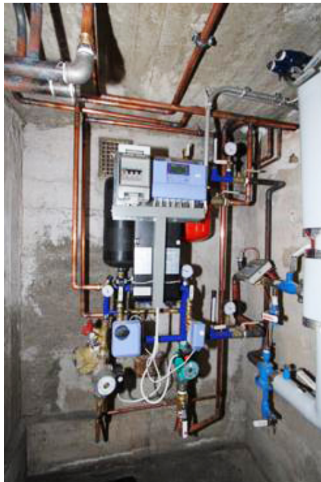
Figure 48. Heat exchange equipment (Rakentaja.fi)
