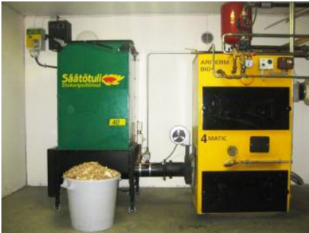
Figure 40. Manually filled stoker burner (40 kW) and a boiler (30 kW), common system for a single family house (0.5 m 3 container)
