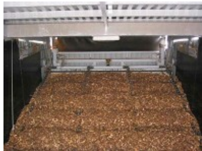
Figure 38. Drag chain unloader (EUBIONET2)
